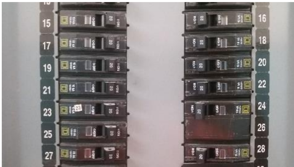
Figure 42: Circuit Breakers (Courtesy of Group 4)
