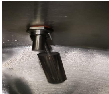
Figure 5: Float Switch (courtesy of Group 4)
